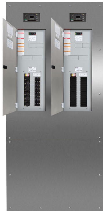
Isolated Power System
