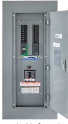
NQ MB Panelboard with SurgeLoc SPD installed
