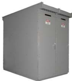
Masterclad 27 kV, Outdoor Non Walk-in, Metalclad Switchgear
